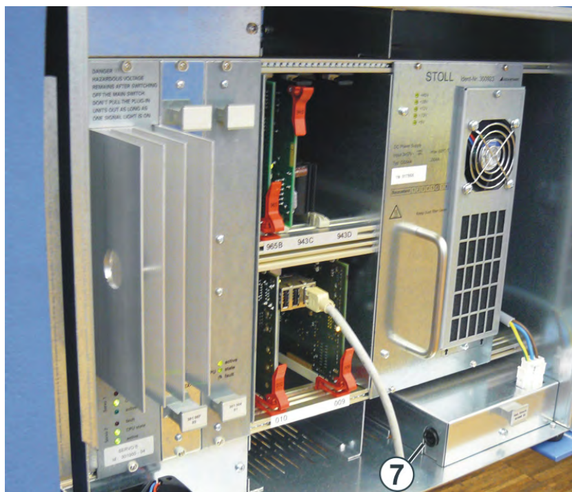
Battery fuse below the power supply unit
