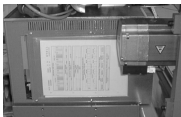
Machine data sheet at the right control cabinet
